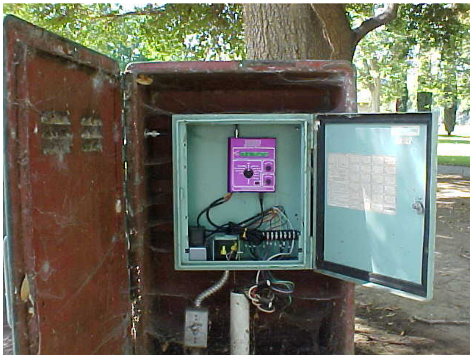
Example of a Hydropoint installation
